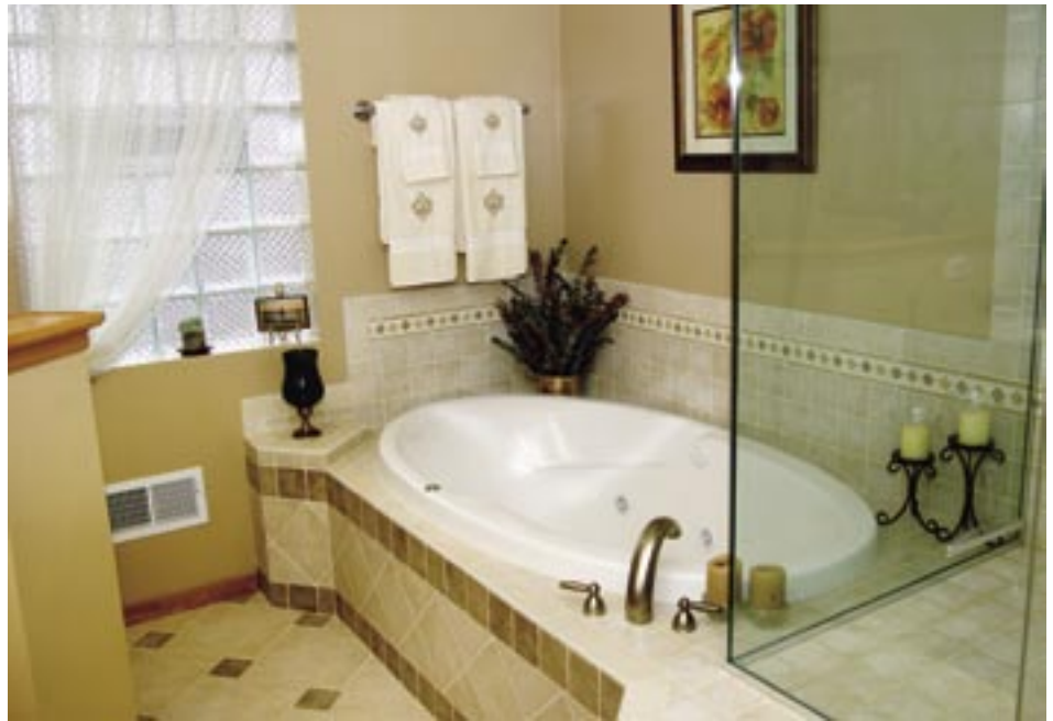
Total bathroom remodel. Whirlpool tub, glass shower enclosure, body jets and rainhead.
